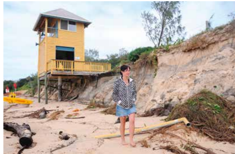
Source 2 A 2009 storm severely eroded the Rainbow Beach foredune, placing the Surf Life Saving tower in danger of collapse.
